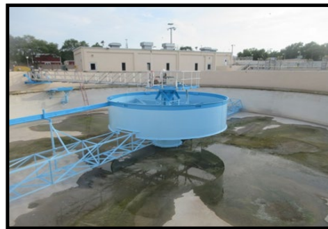
Wastewater Treatment Plant- North Clarifier
