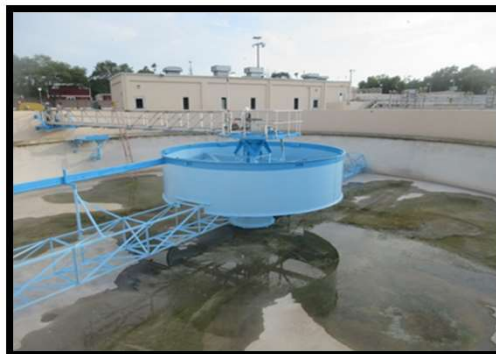
Wastewater Treatment Plant- North Clarifier
