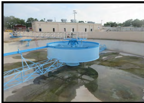
Wastewater Treatment Plant- North Clarifier
