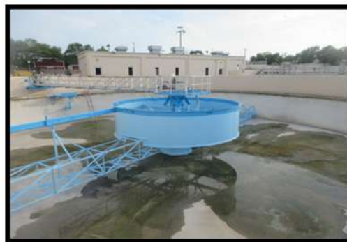
Wastewater Treatment Plant- North Clarifier
