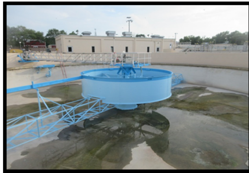
Wastewater Treatment Plant- North Clarifier
