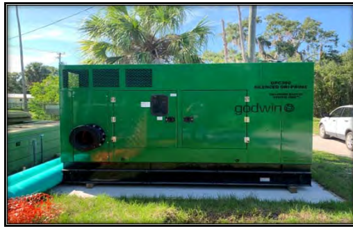
Pictured above - City of Dunedin , Lift Station #8 Standby Emergency Pump
