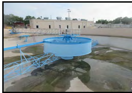
Wastewater Treatment Plant- North Clarifier
