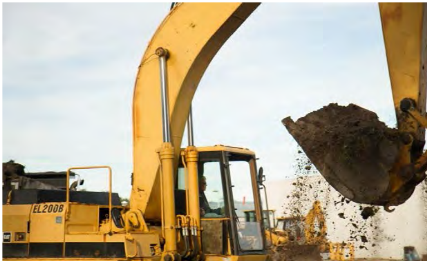
Stormwater scheduled maintenance
