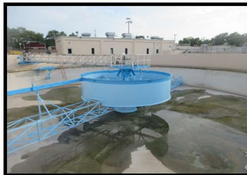
Wastewater Treatment Plant- North Clarifier
